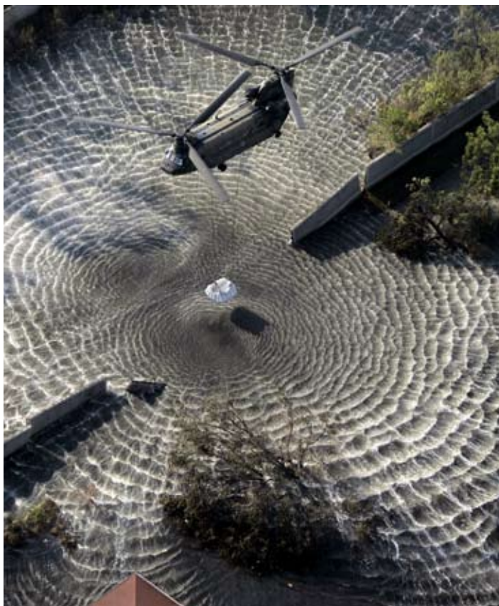
■ SEPT. 4, 2005: A helicopter lowers a sandbag into the broken section of a New Orleans levee.
