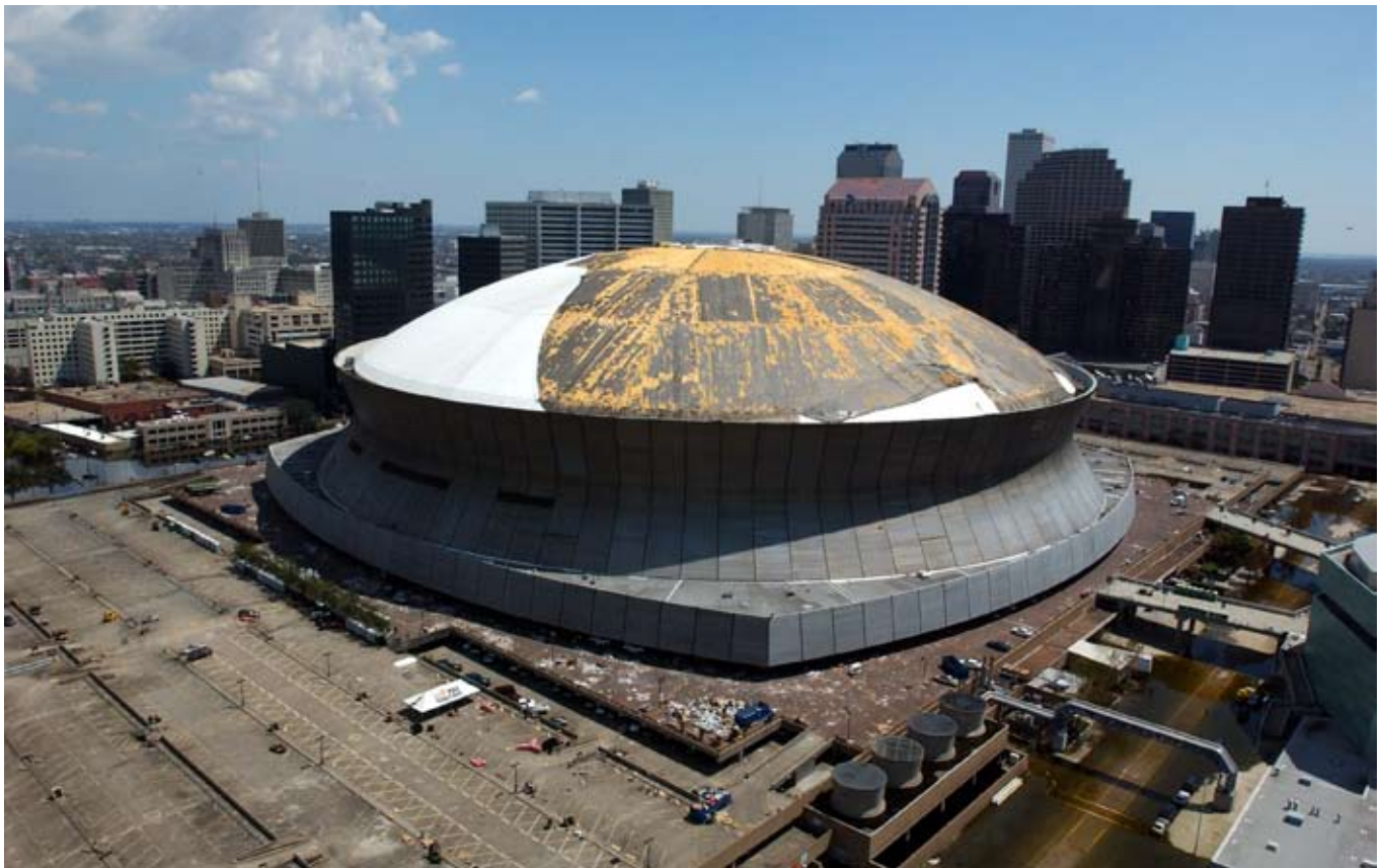
■ NEW ORLEANS, SEPT. 8, 2005: The roof of the Superdome was battered and stripped by the destructive winds of Hurricane Katrina.
