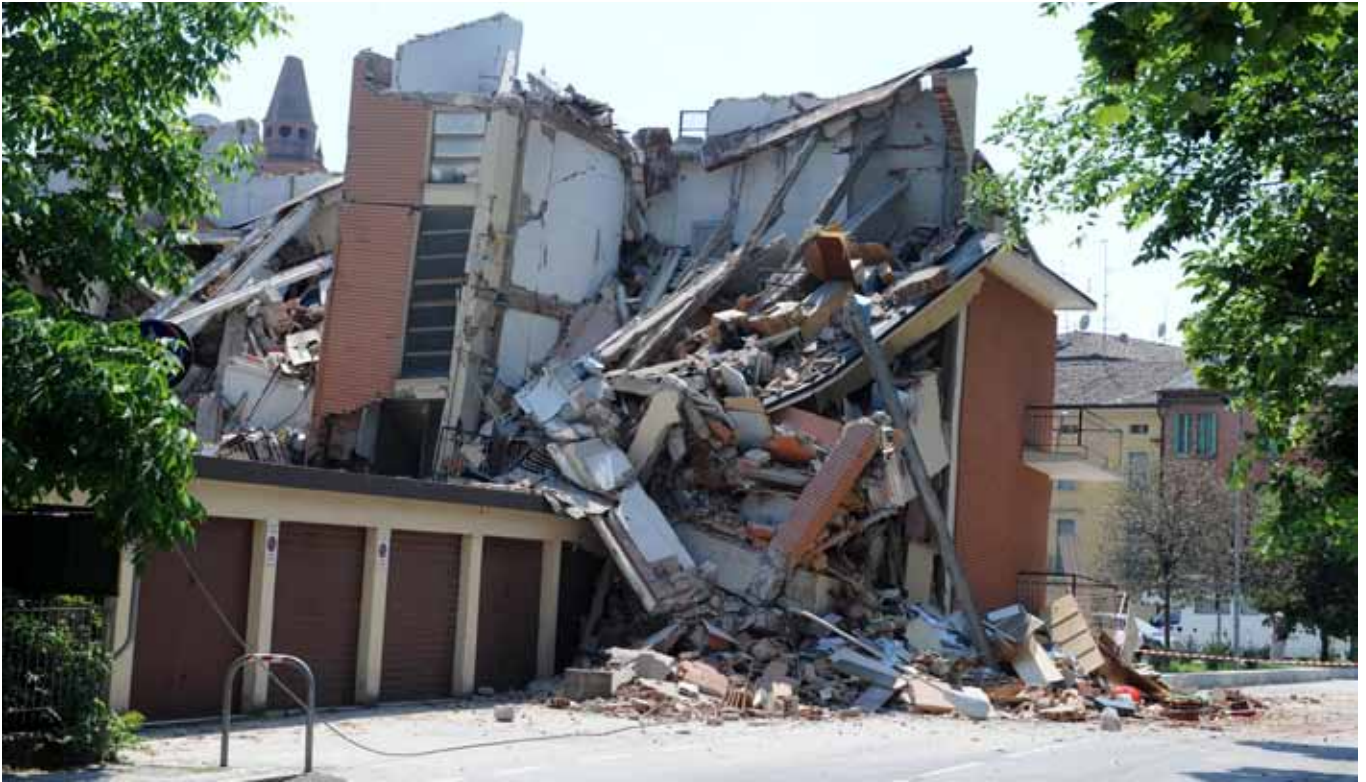
■ COLLAPSE: A building is damaged after an earthquake in Cavezzo, Italy (May 29, 2012).
