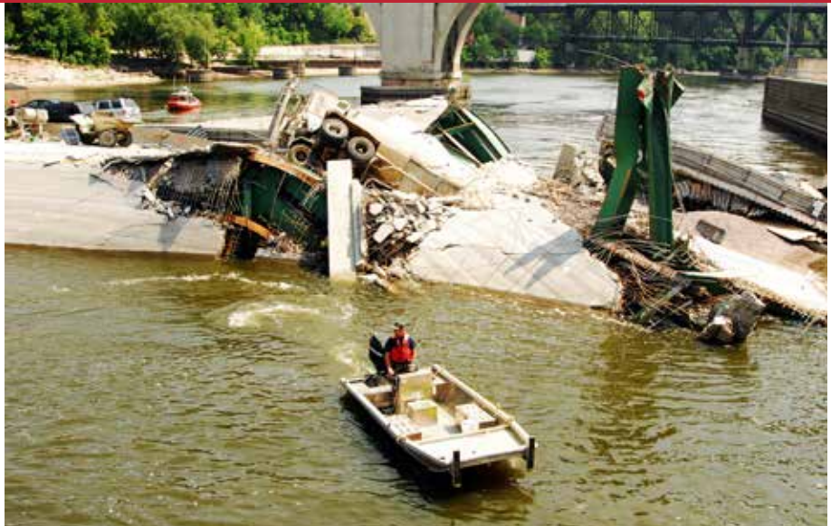
■ DEADLY FAILURE: Navy divers survey and assess the wreckage of the I-35W bridge collapse in Minneapolis, Minnesota (August 7, 2007). The tragedy, which killed 13 and injured 145 people, is one of the most well-known examples of failed infrastructure.
