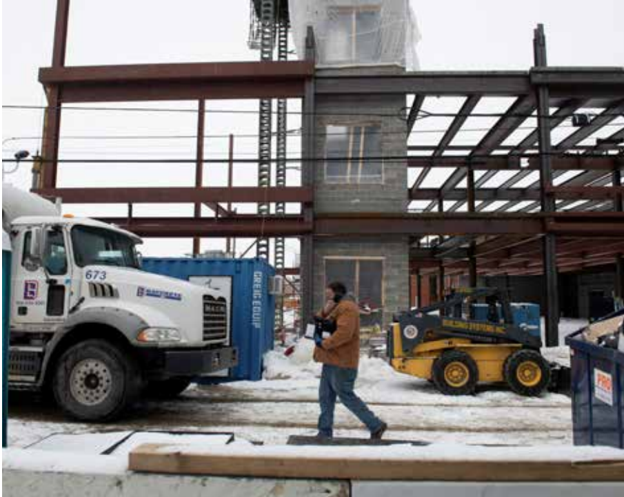
Workers finish the day at the site of new mixed-use construction in downtown Erie, Pennsylvania, where city leaders are hoping to get a piece of the $500 billion promised through President Biden's infrastructure bill to continue their vision to revitalize their downtown and waterfront areas, moving the city forward from its industrial past (Feb. 8, 2022).
