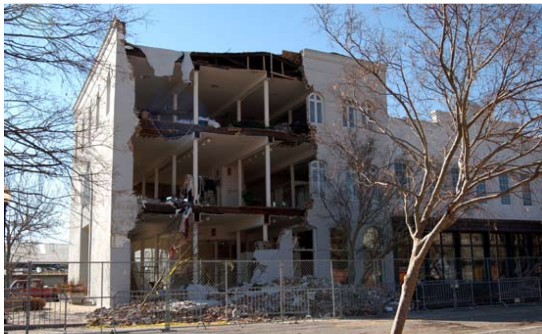
■ DOWNTOWN DESTRUCTION: Some downtown Pensacola, Florida structures like this one were severely damaged by Hurricane Ivan (Oct. 12, 2004).
